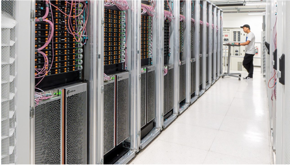
A Cerebras Supercomputer Deployment at One of Our Colocation Facilities
